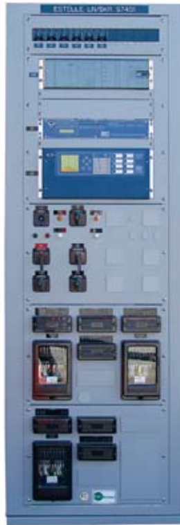
Line Breaker Panel
