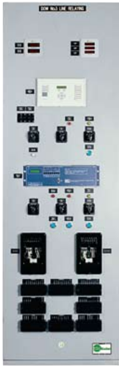
Line Breaker Panel
